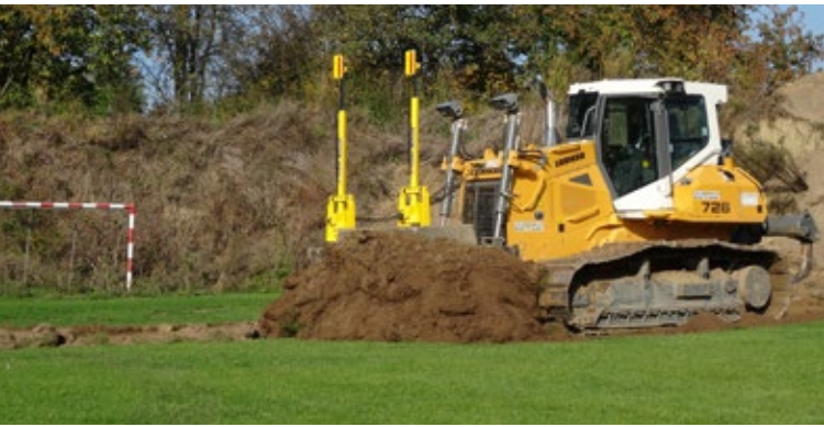
Sports field refurbishment: precise removal of the lawn layer using 2D laser control
